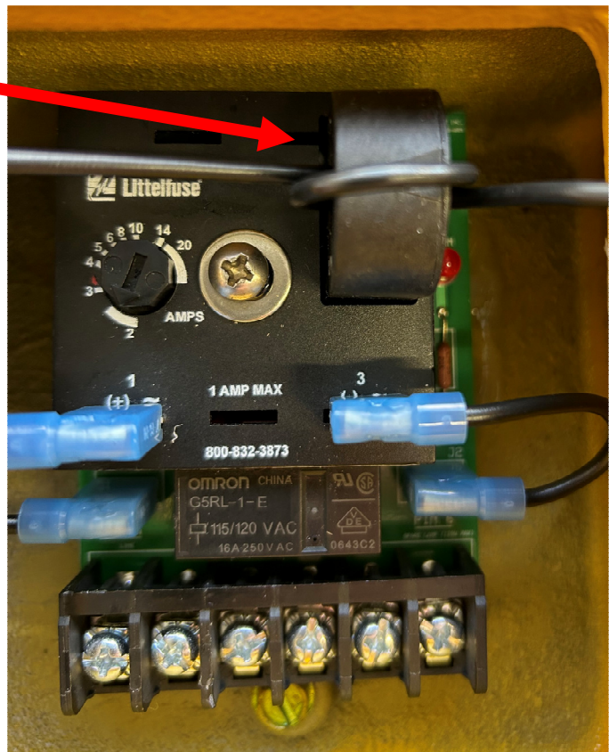
PHOTO 1 (Incandescent Light Fixture Toroidal Transformer Wiring)
