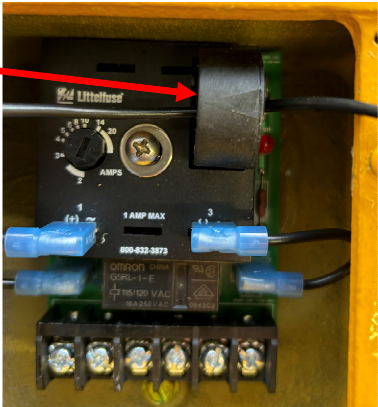
PHOTO 2 (L-864 Beacon Toroidal Transformer Wiring)
