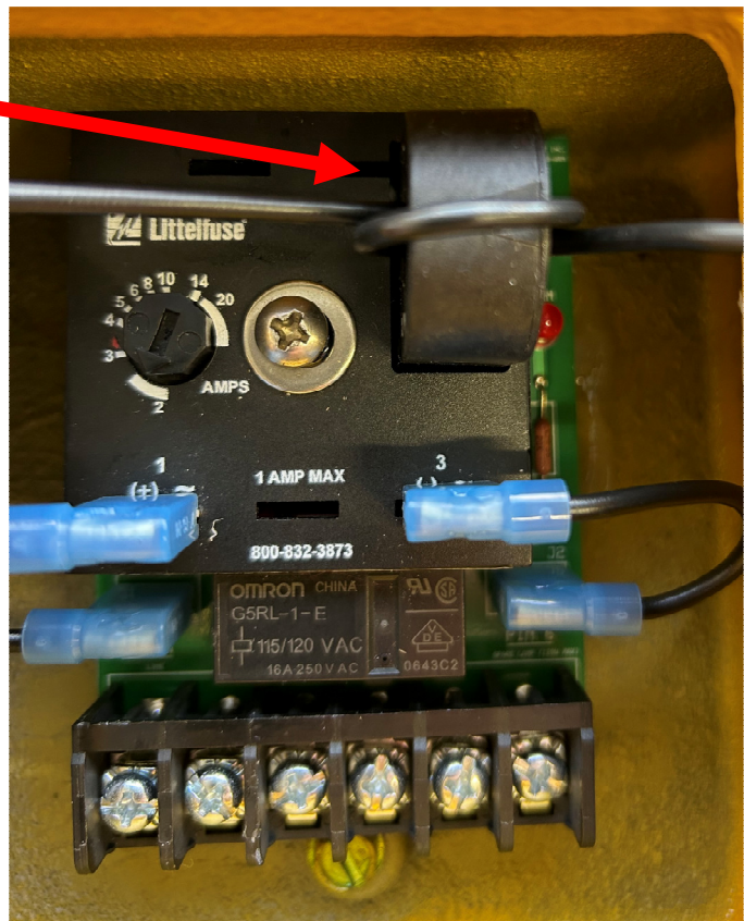
PHOTO 1 (Incandescent Light Fixture Toroidal Transformer Wiring)
