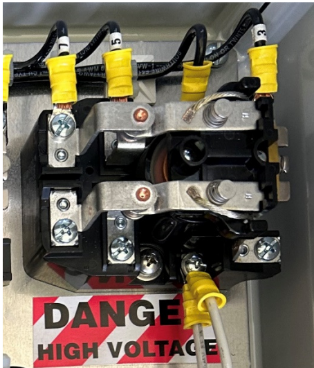
External Contactor Relay
